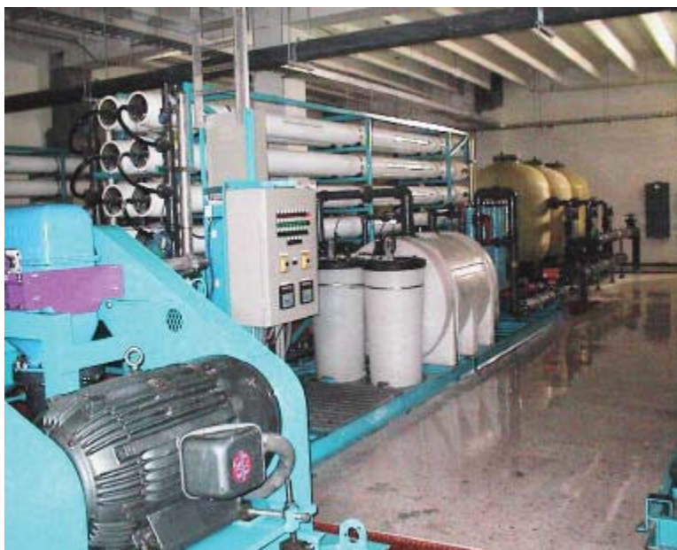
Fig. 2: An example of the Reverse Osmosis (RO) purification equipment used in the PS
