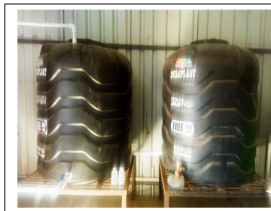
Fig. 4: Treated water tanks inside the EDF plant
