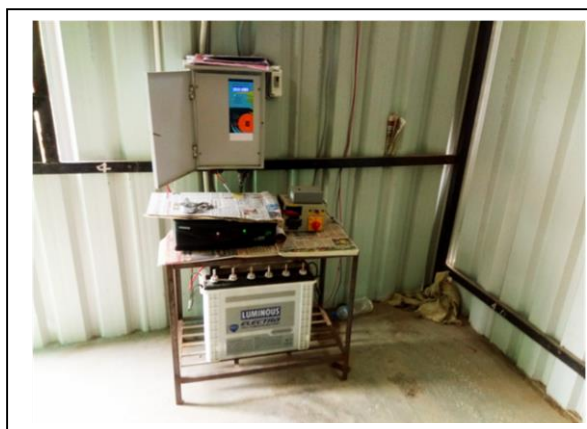
Fig.1: Charge controller, battery inverter, DC regulator & battery (200 AH) inside EDF plant
