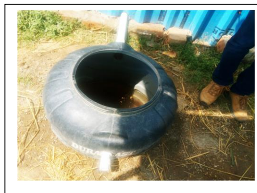
Fig. 6: Sludge collection unit provided outside the EDF plant
